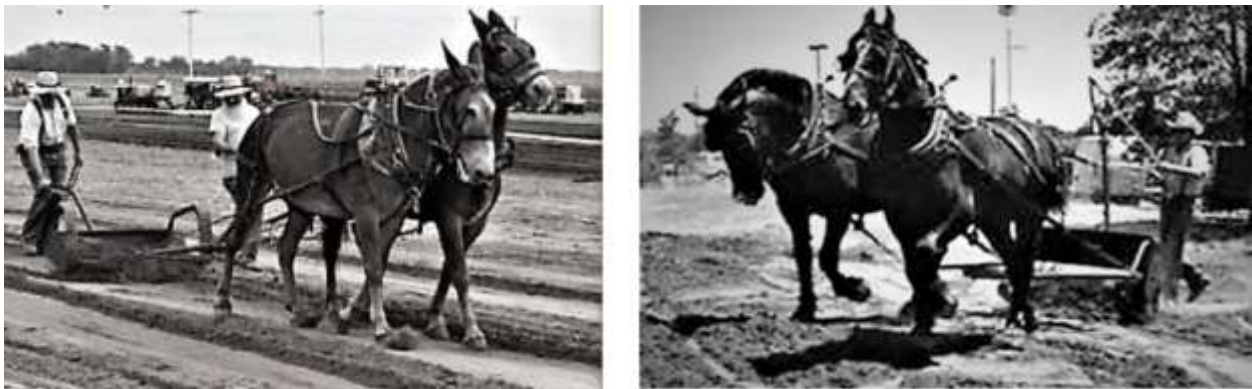
Figure 26 Left: Muleskinners operate a Fresno Scraper to scrape soil into the scraper's bucket. Right: An individual Fresno Scraper operator has tilted the handle upright to empty the Fresno Scraper's load.
